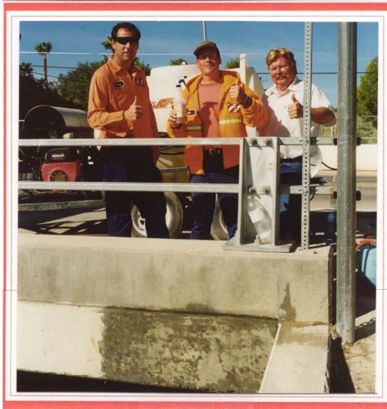
TAGINATOR® removes multi-layered spray paint graffiti from pre-cast concrete. ( Clark County, NV )
