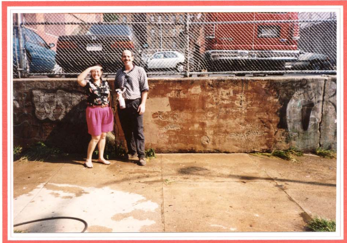
TAGINATOR® removes spray paint graffiti from old patched concrete. ( New York, NY )
